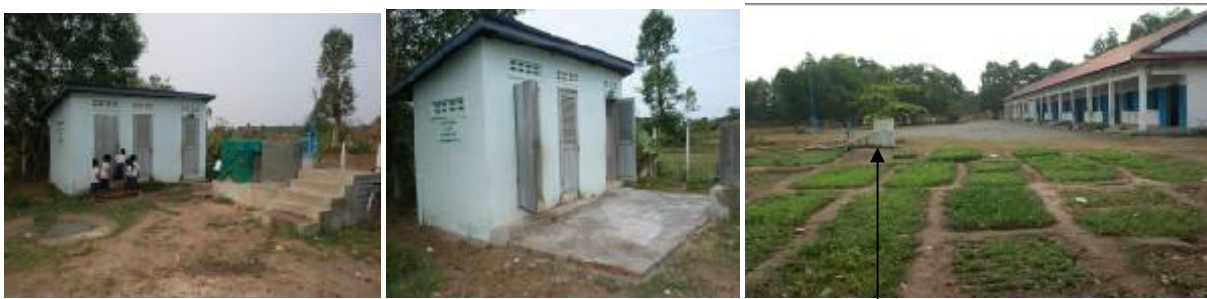
1 three-room latrine in Khvien primary school was repaired and re-opened for pupils and teachers
