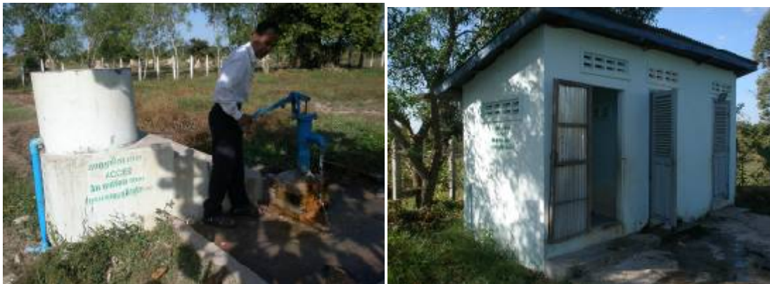
1 well and 1 three-room latrine in Khvien primary school were repaired and re-opened for pupils and teachers
